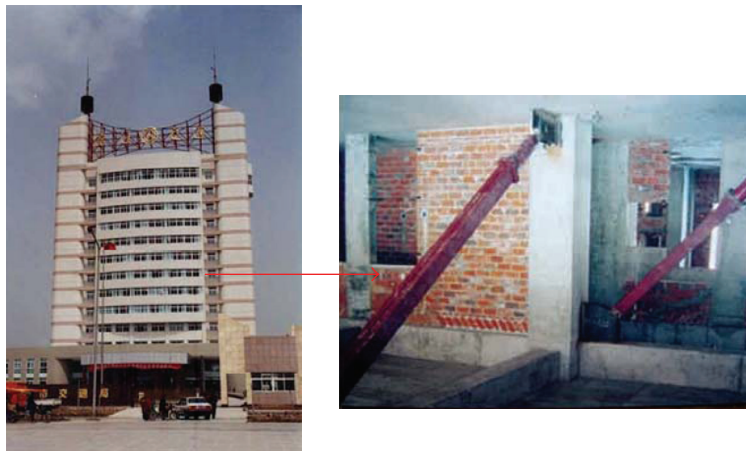
Figure 9: Viscoelastic dampers in Suqian Communication Building.
